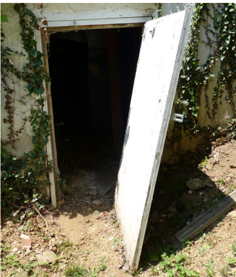
Basement Door, CPG, July 2024
